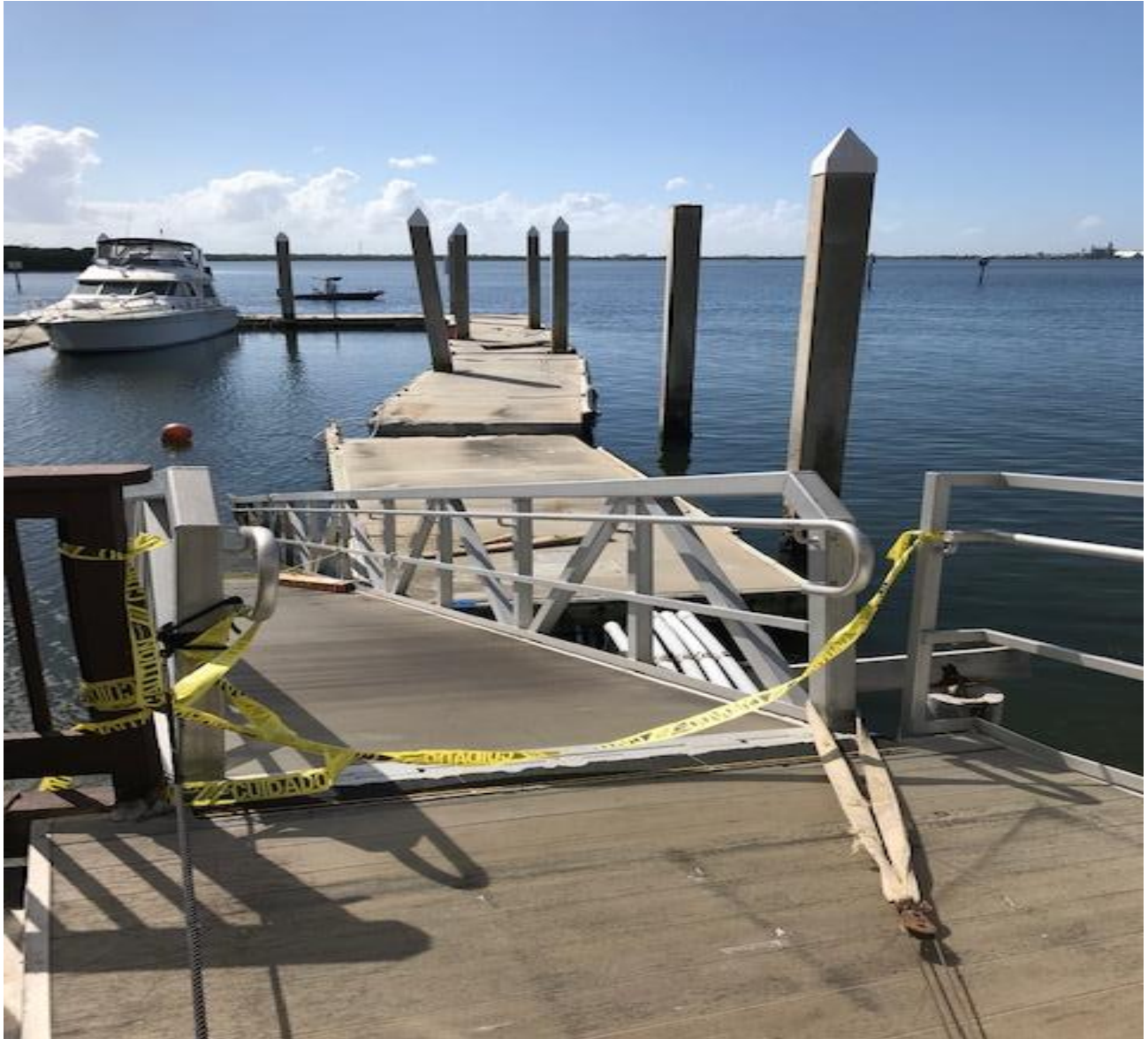
Storm damage to waler-style concrete docks, gangway, and utilities
